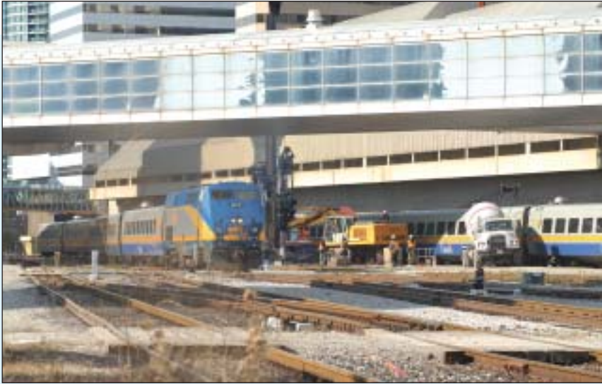
LoDril and IMT drilling at the Simcoe Extension project. Note restricted working area between trains for drilling and placing concrete.
