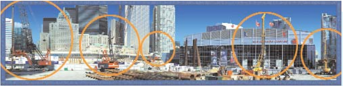
Drilling caisson walls and structural caissons with crane mounted and track mounted drilling equipment at the Maple Leaf Square and TELUS sites.
