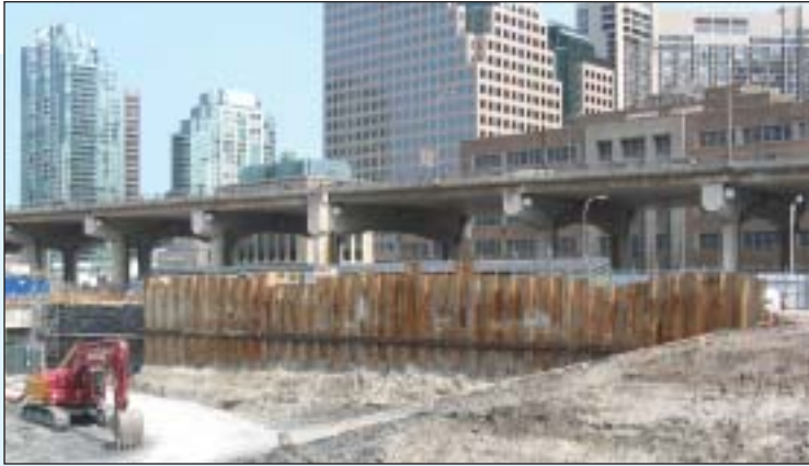
Installation of temporary sheet piling and rock anchors along the south wall is complete. Excavation is continuing.
