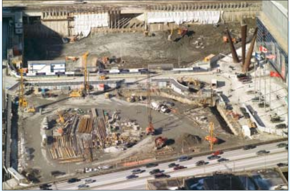
Overview of Maple Leaf Square site (bottom) and TELUS site (top), Air Canada Centre (right). Anchor Shoring was the contractor on all three projects.
