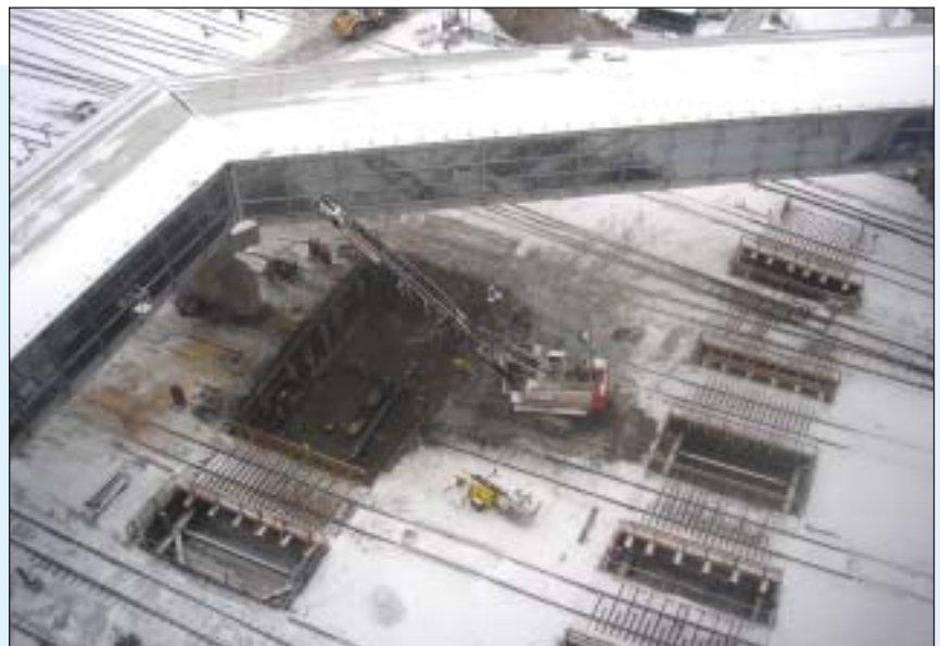
Aerial view of track level at the Simcoe Street Extension. Trestle installation work underway. Five trestle bridges are complete.
