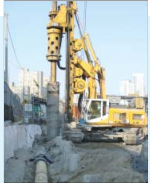
Anchor drilling adjacent to live gas main with a BG24H for the south caisson wall.
