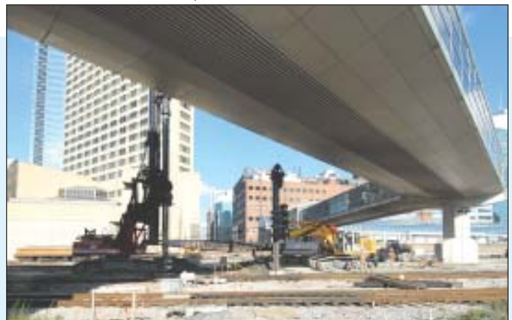
Drilling soldier pile holes at track level for the Simcoe Extension project. A LoDrill is working below skywalk. An IMT is drilling for piles in areas with unrestricted headroom.
