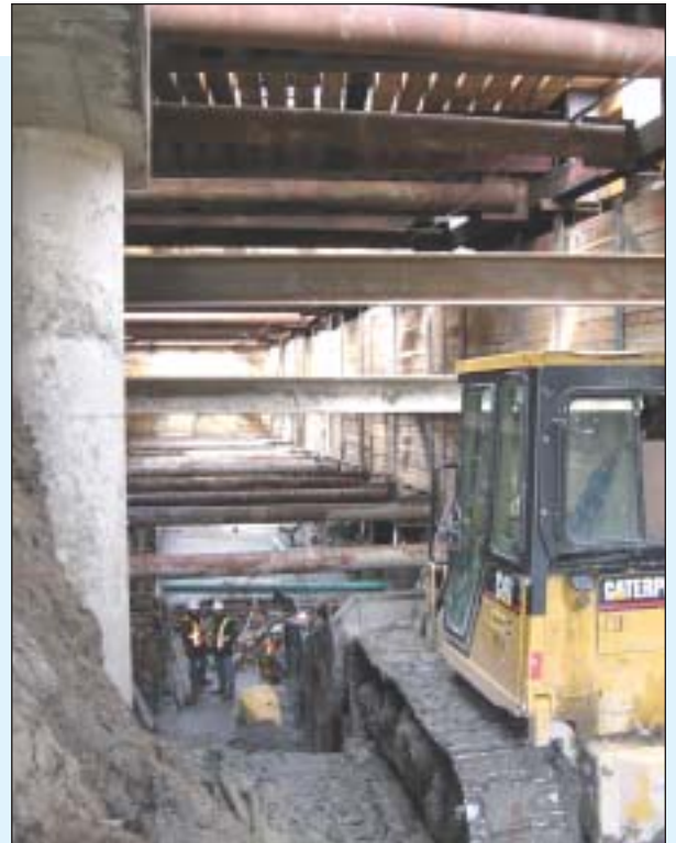
Three rows of struts have been installed to brace the shoring walls. Excavation continuing to top of shale bedrock.
