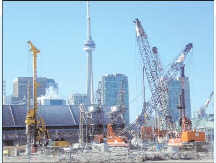
Installing caissons at the Corus Entertainment Headquarters with a Bauer BG28H, a Hain drill mounted on an LS208 crane, an IMT AF180 drill rig and associated support equipmen
