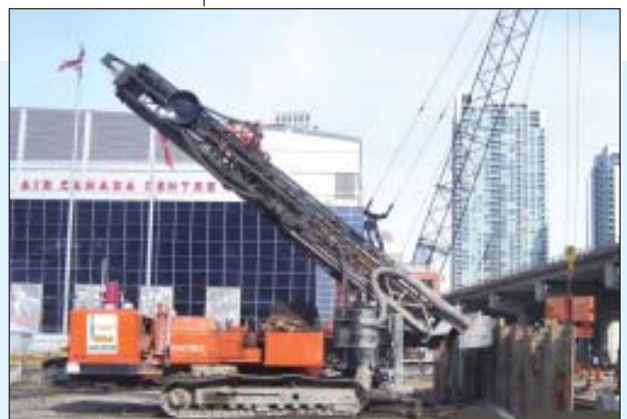
Installation of rock anchors by Crown Drilling to brace the south sheet pile wall at Maple Leaf Square.
