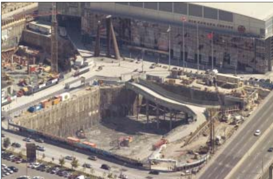
Aerial view of completed caisson walls, rock protection, temporary ramp, sheet piling and drilling of south caisson wall at the Maple Leaf Square Project.
